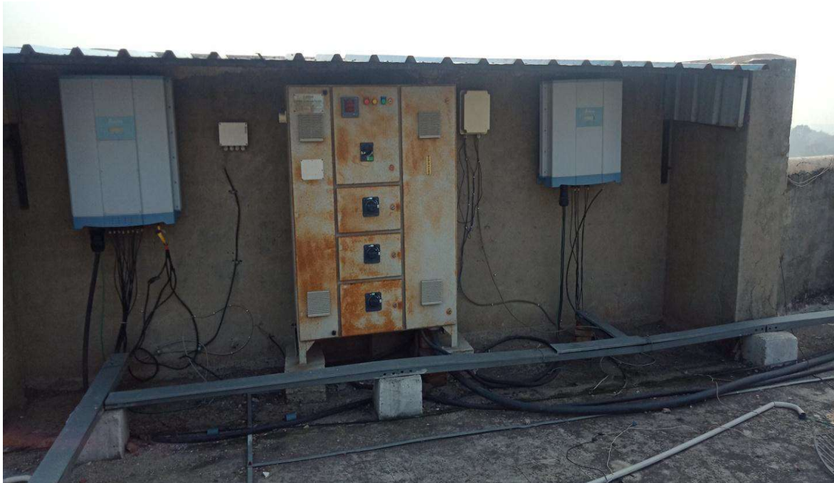
Photo: Output control panel of the Solar Power System
